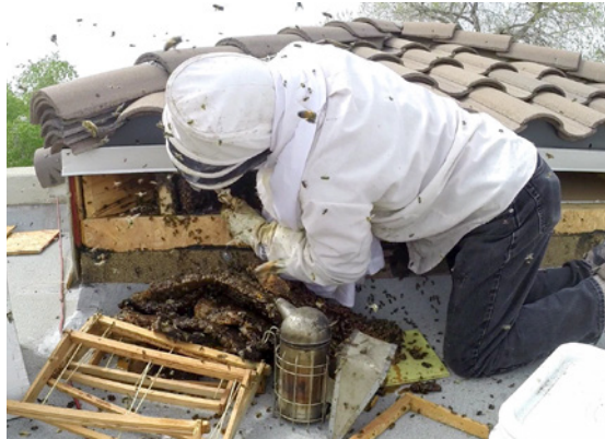
A poorly repaired cable installation allowed a swarm to take up residence in this Four Hills home.
